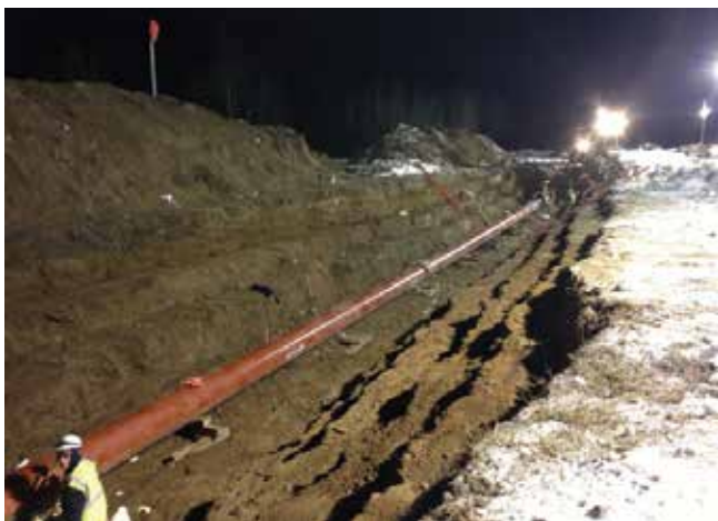
Figure 5. 150' of pipeline removed from service due to sediment levels.
